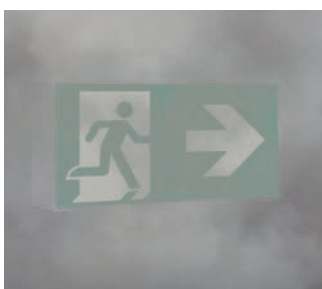
Badly illuminated escape sign
